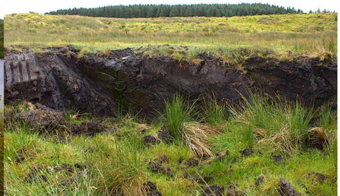
the road from the forestry towards T12 T13 and T14 would cross this area of what appears to be wet grassland but can be seen to be 2m deep peat !
